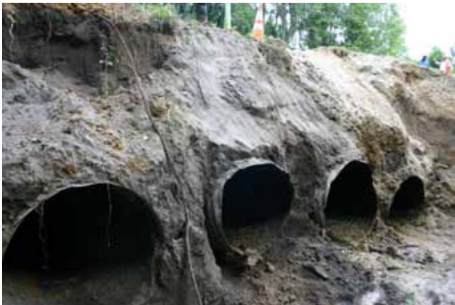
The culvert consisted of four badly corroded pieces of corrugated metal pipe in a row.
