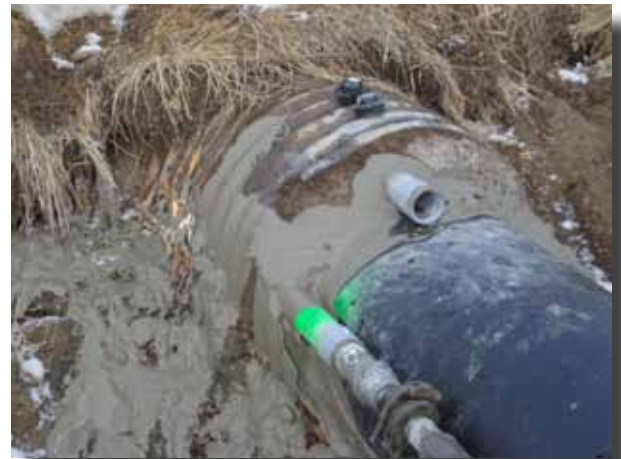
Grouting, filling in the space between the new liner and old culvert
