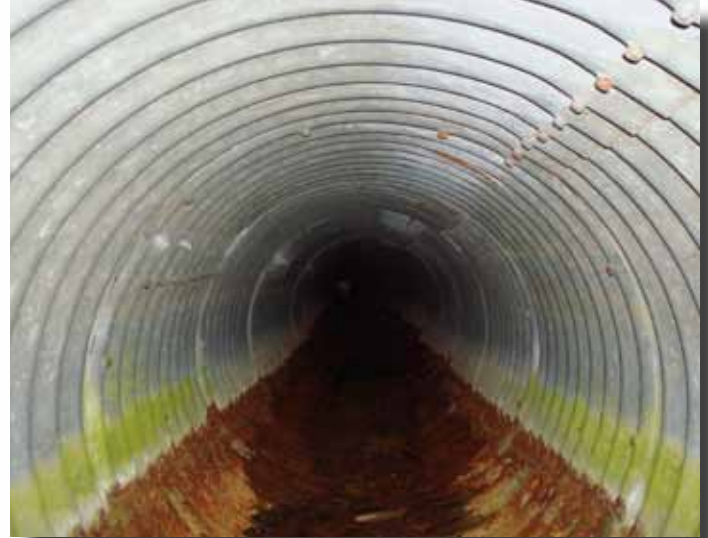
Culvert inspected in the fall, showing invert corrosion after cleanout
