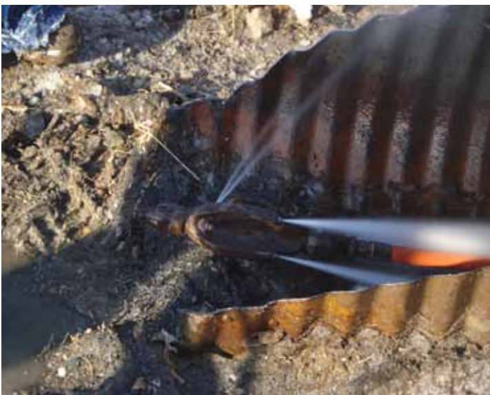
Winter cleanout of culvert using heated water in a rodder/jet hydrovac truck
