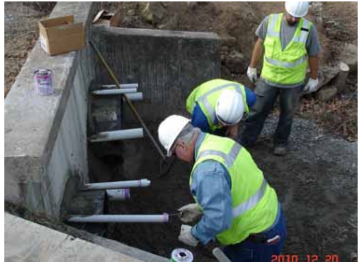
Any space between the old CMP and the new Snap-Tite liner is filled in with grout.
