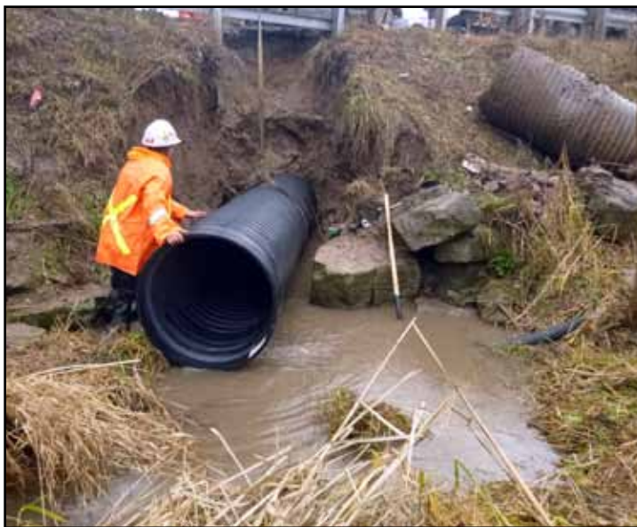
A view of the worksite from the upstream side. A piece of the failed CSP is removed and on the right side of the picture.
