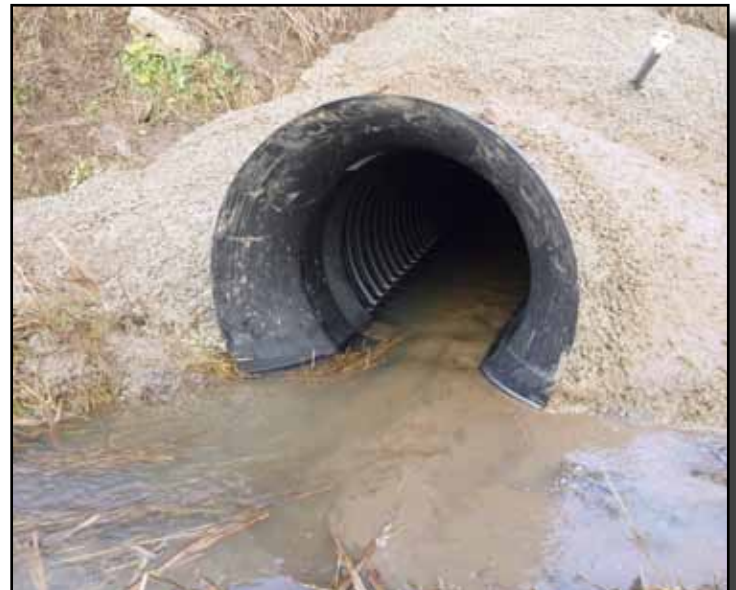
A view of the upstream side of the IOP pipe with the Hydro-Bell attached, after the project is completed.
