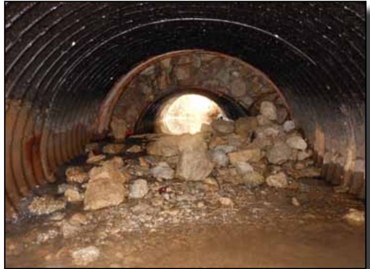
A view inside the failing structure at the joint.
