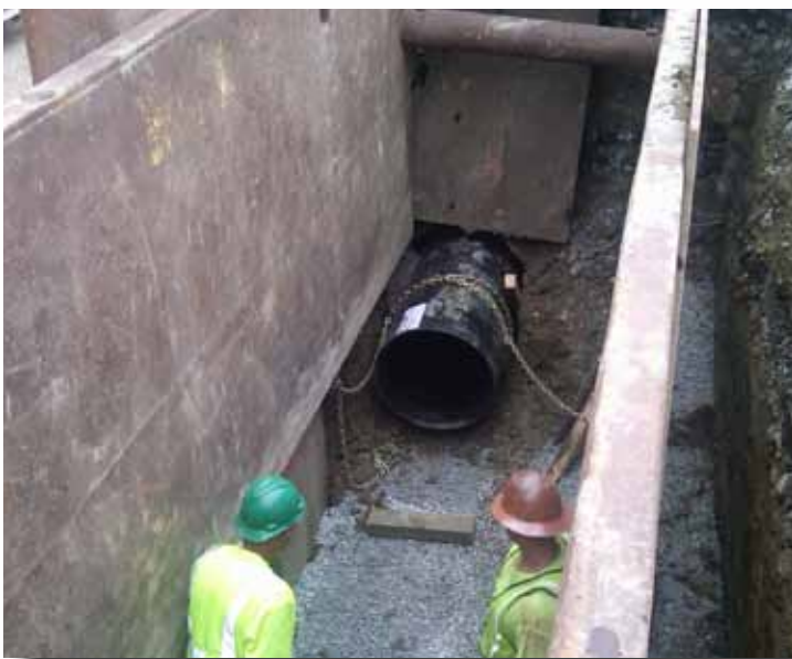
The Snap-Tite® pipe section is pushed inside the old culvert and then will be snapped to another end of Snap-Tite® pipe using only a come-along and chains.
