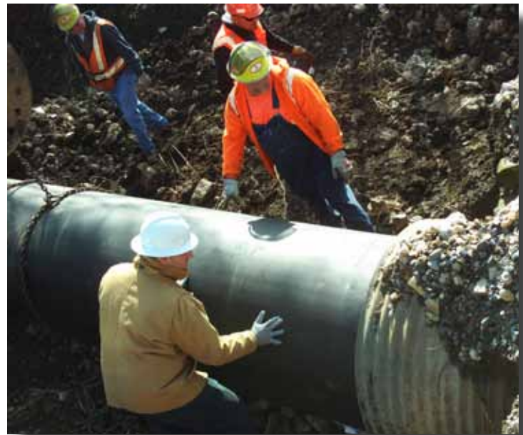
Union Pacific was able to use its own crews to install the Snap-Tite pipe without needing to hire outside contractors.
