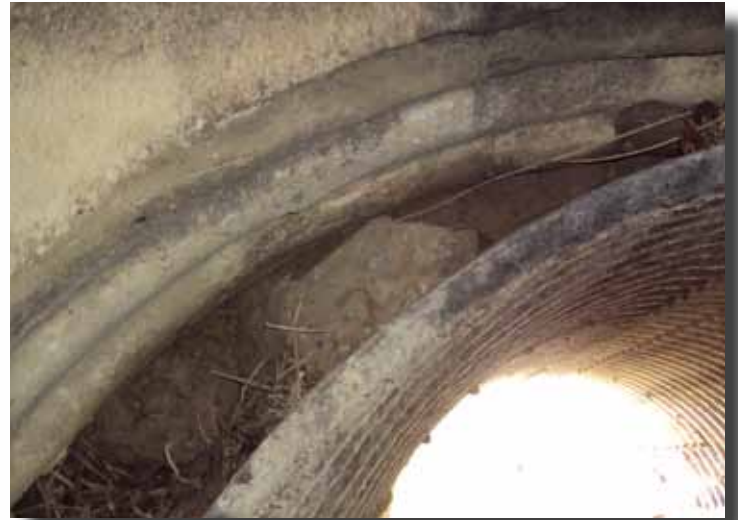
The old levee culvert was damaged and failing in several areas of the length of the pipe. Flooding was a concern.
