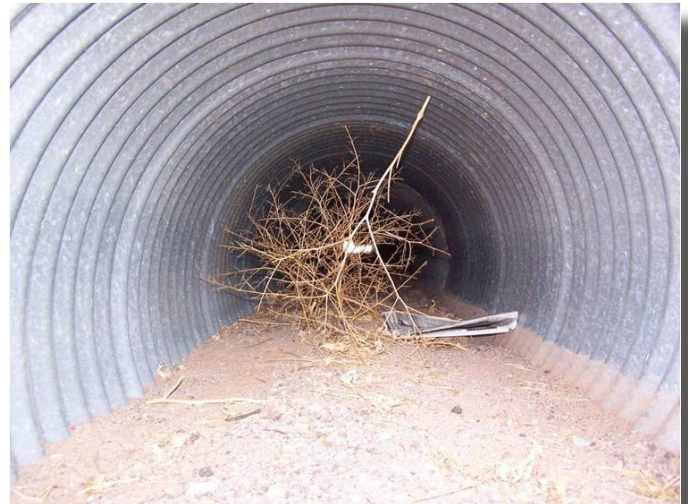
With 8" – 10" of sediment inside the 30" CMP, the culvert had to be cleaned prior to installation of 24" Snap-Tite pipe.
