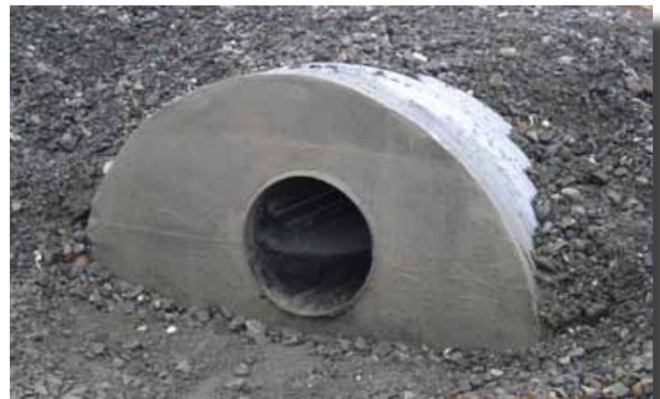
The installation is complete. The culvert is lined with Snap-Tite® pipe and the annular space is filled in with high-pressure grout.
