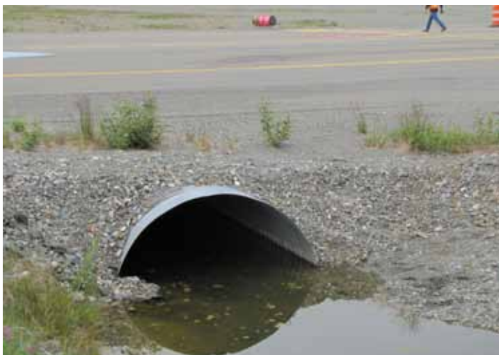
The CMP buckeling under the pressure of the traffic on the taxiway.
