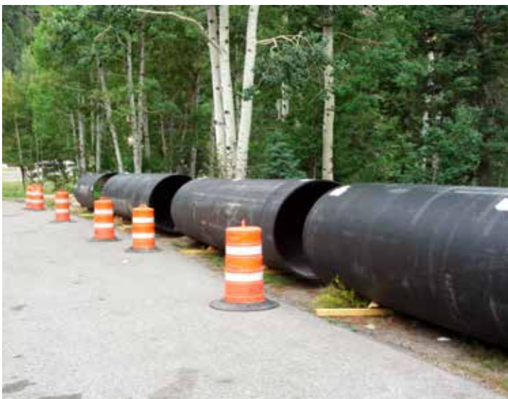
Sections of Snap-Tite HDPE pipe awaiting installation on the side of the road.
