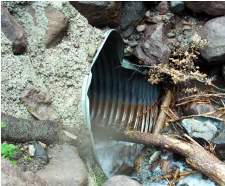
One of the damaged culverts before it was repaired.
