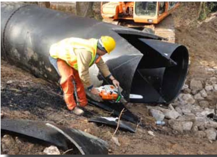
A DOT maintenance worker cuts a bullet nose on one end of a Snap-Tite® pipe section.
