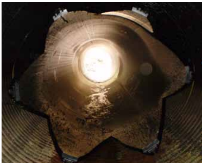
The bullet nose Snap-Tite® end of the pipe is slid through the deflected old culvert.
