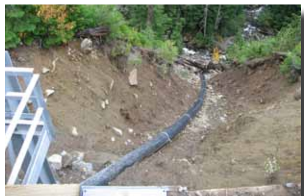
Figure 5: The down-slope pipe.
