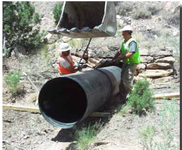
The Snap-Tite pipe is pushed inside the old culvert. Once the snapped liner is slid in place, any annular space between the liner and culvert is filled in with grout.
