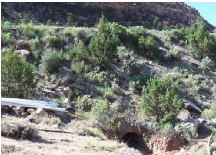
Here is an example of the 60-feet of deep fill (cover) over the wood culverts that was too cumbersome to dig.
