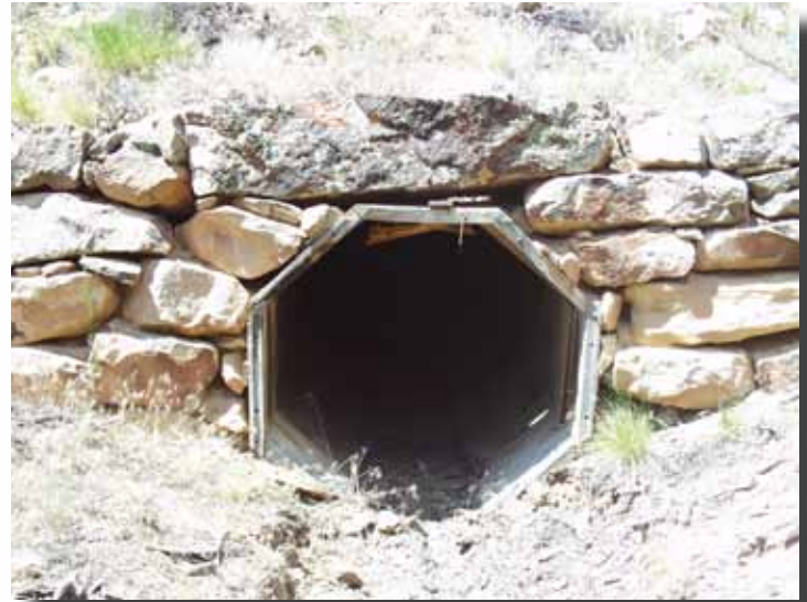
One of the octagonal wood culverts installed in the 1920s. This one measured 36 inches in diameter.
