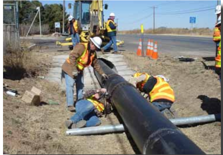
DOT maintenance crew snaps the culvert liner pipe together with come-alongs and chains.
