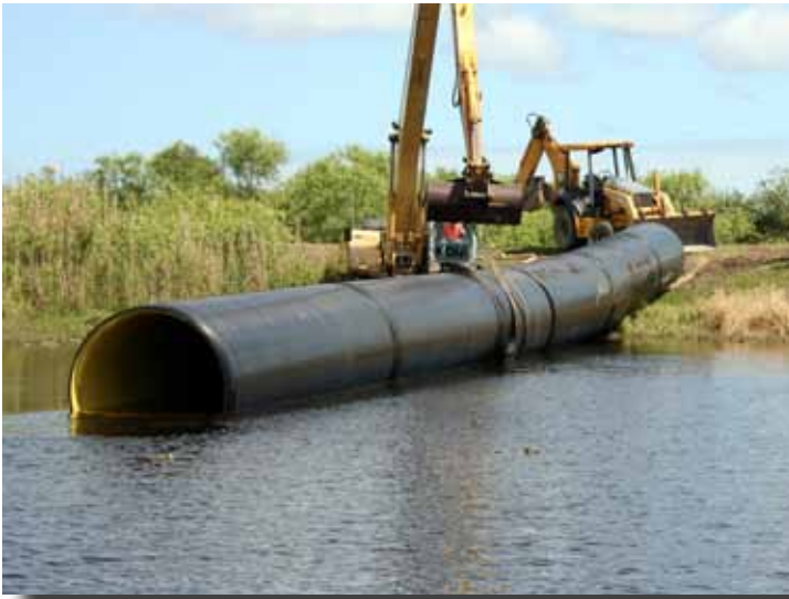
The electrofused PPT pipe was placed in the water to be submerged under water and pushed into the old pipe.
