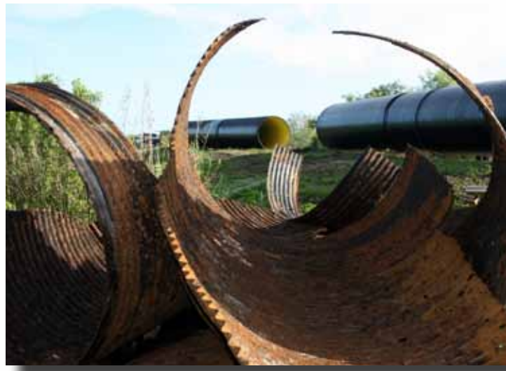
A view of the excavated deteriorated corrugated metal pipes with the new profile wall pipe liner in the background.
