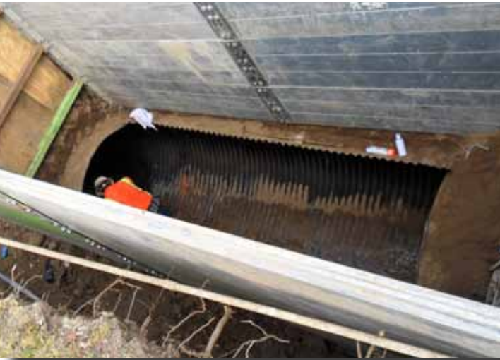
The pit where the deteriorated culvert needed to be relined.
