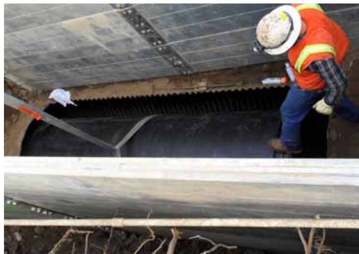
A pipe liner section is pushed through the old existing pipe so that another Snap-Tite® section can be snapped together.
