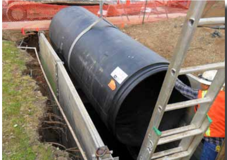
Snap-Tite® pipe is lowered into the pit in order to reline the old CMP culvert.
