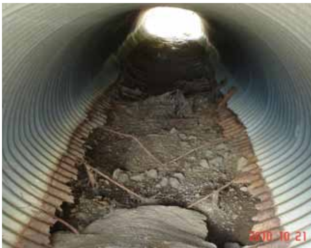
Before: the damaged CMP before it is relined.
