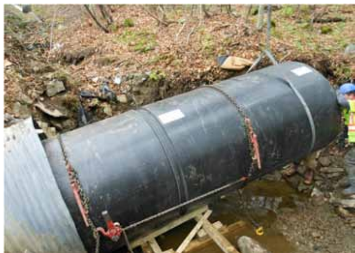
The snapped sections of pipe are slid inside the old CMP, completely lining the deteriorated pipe.
