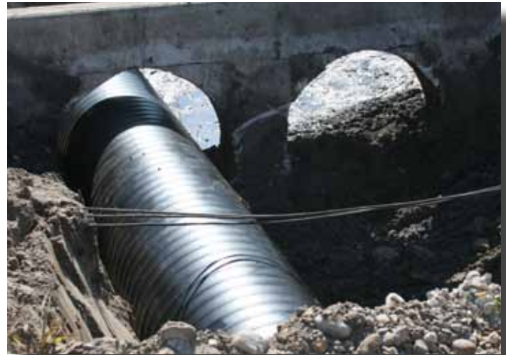
The closed profile pipe is pushed through to reline the other damaged culvert, without having to replace the headwall.
