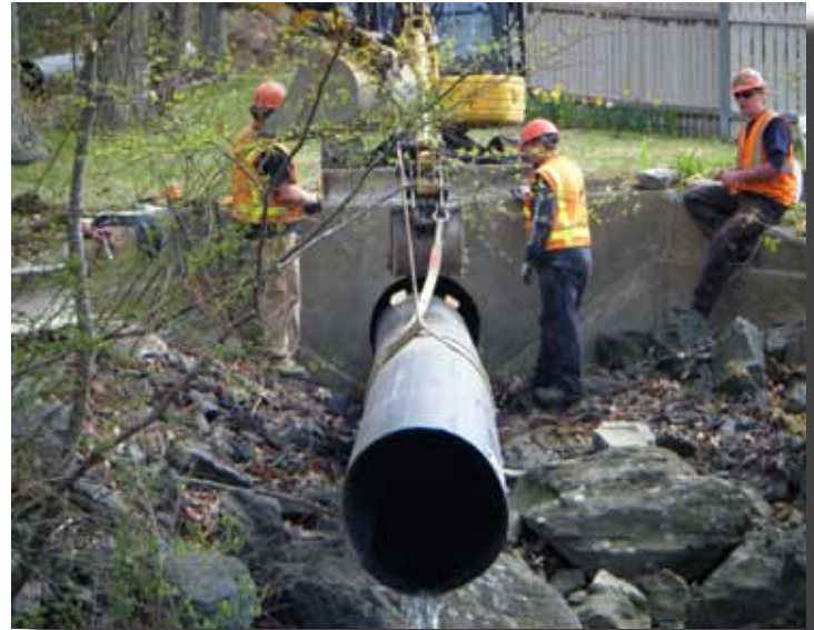
Snap-Tite pipe is slid inside the old storm drain. Relining the pipe is quicker and safer than a dig and replace method.
