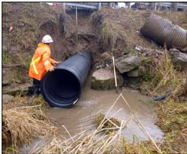
A view of the worksite from the upstream side. A piece of the failed CSP is removed and on the right side of the picture.
