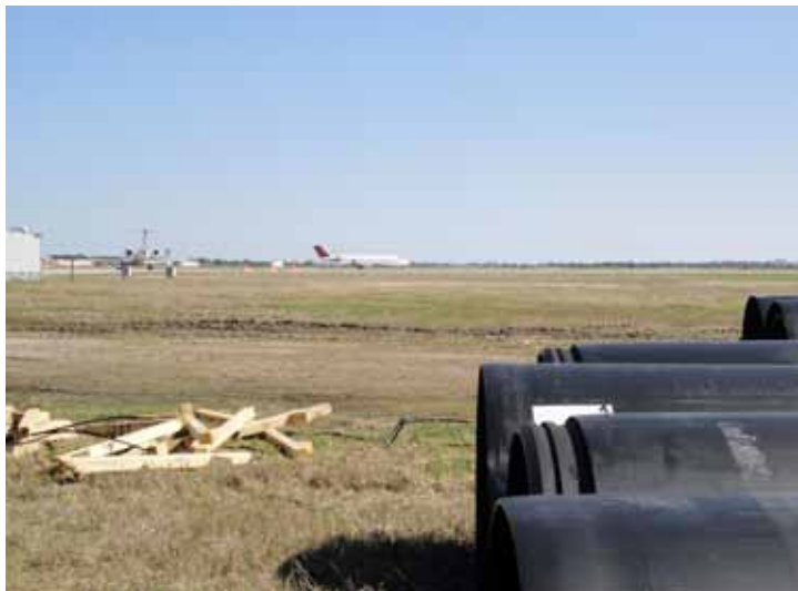
The runways and taxiways remained operational during the culvert relining phase of the project.
