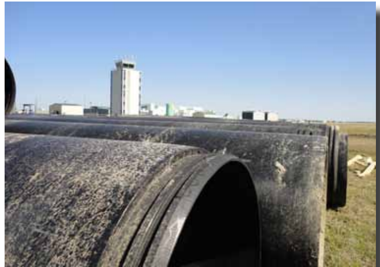
The machined ends of the Snap-Tite pipe are joined together using come-a-longs and chains. Then, they snapped sections are slid inside the old culvert.
