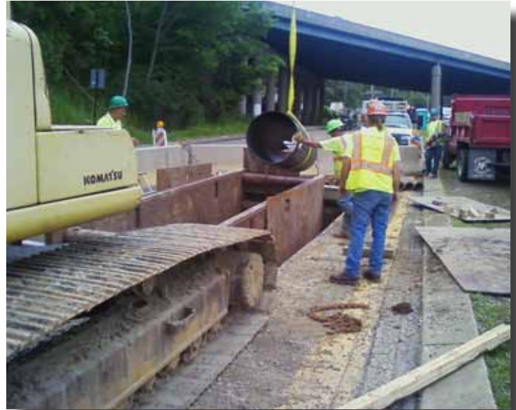
One section of the Snap-Tite pipe is lowered down to begin the reline process.
