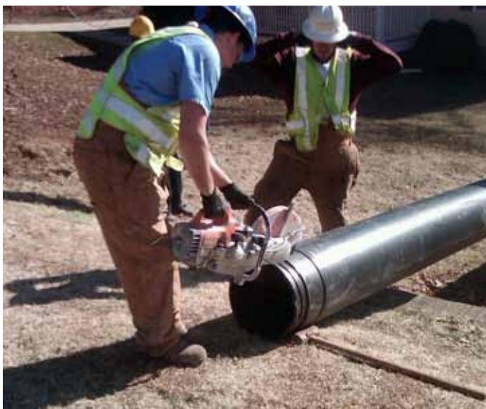
The city's crew cuts a bullet nose into one end of the 18-inch Snap-Tite pipe liner in order to slip the liner into the deflected old CMP culvert.
