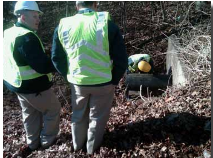
Jimmy Lineman, Gastonia's public works engineer (pictured on the left), observing the installation on site.
