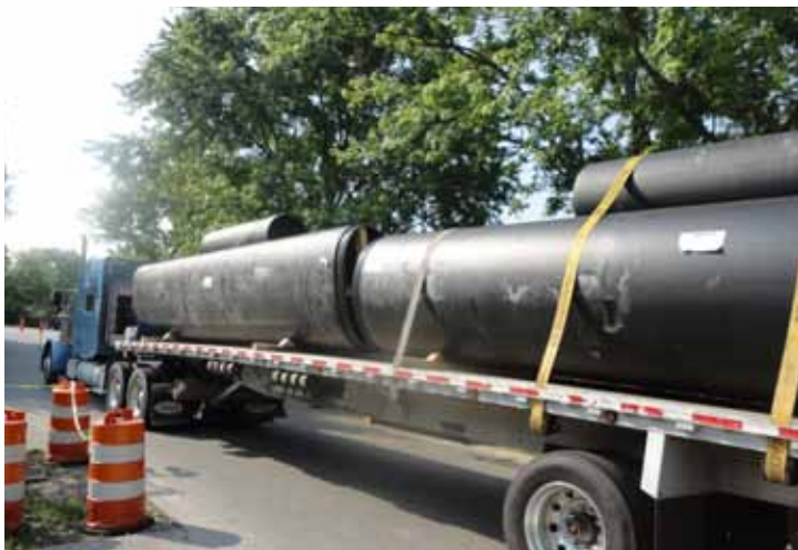
Snap-Tite supplied sections of ovalled Snap-Tite HDPE pipe to line the oval culvert. Snap-Tite delivered a total of 190 feet of pipe.
