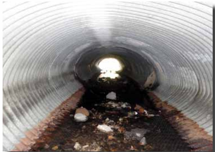
The original culvert was corroded and in bad shape. It was located in a residential neighborhood so if it failed it could compromise the foundation of some homes.
