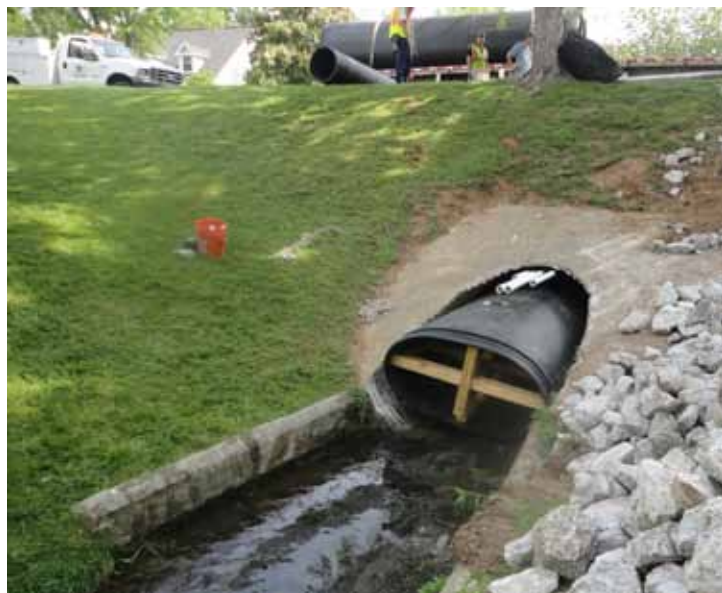
The Snap-Tite pipe liner was slip-lined into the old culvert one section at a time. Each section was snapped together using a come-a-long and chains.
