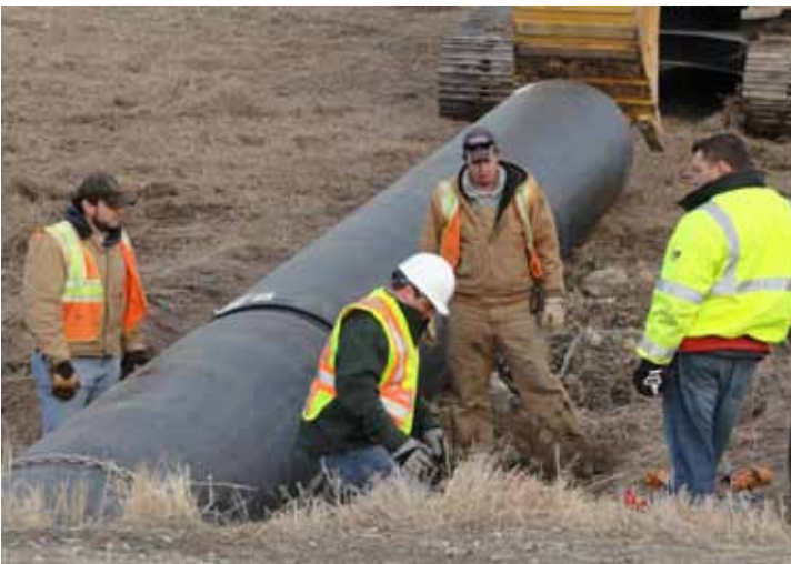
One section of the liner is first inserted into the CMP and then snapped to another section.
