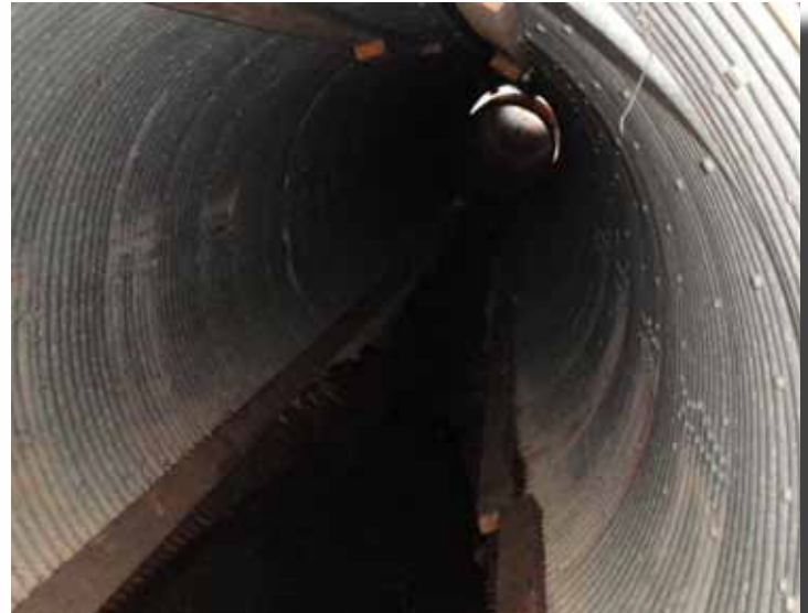
Inside the old CMP culvert, showing signs of wear and deflection.
