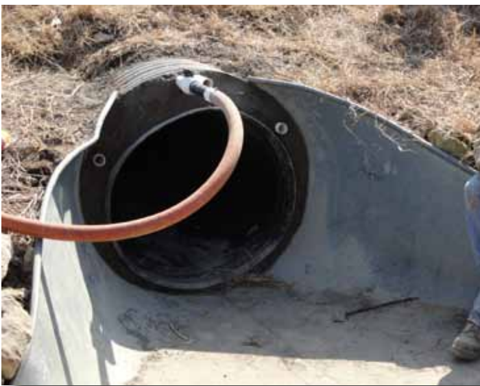
Grout is pumped in to fill in any voids in the annular space between the liner and CMP.
