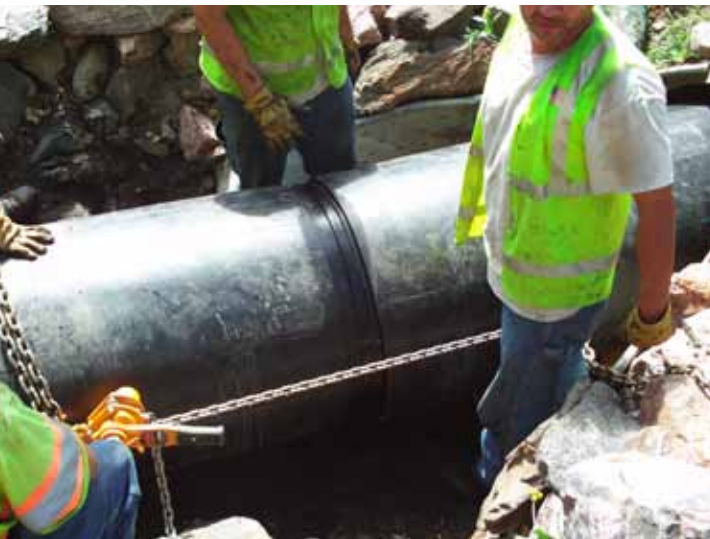
SEMSWA crews join the Snap-Tite pipe sections using a come-along and chains.
