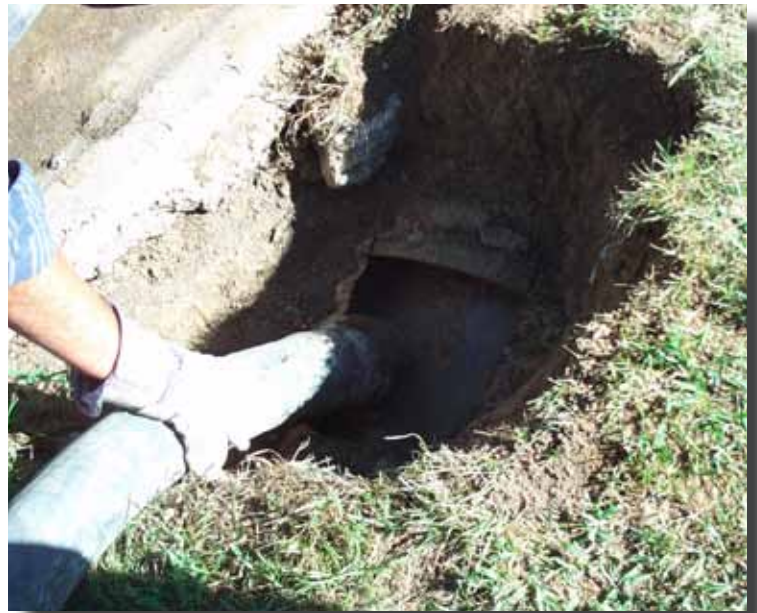
Any annular space between the old CMP and the Snap-Tite pipe liner is filled in with grout.
