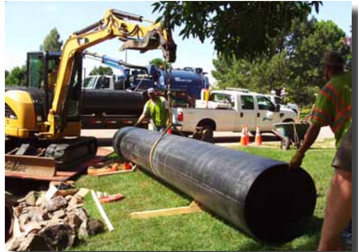
The Snap-Tite pipe is moved in place to line the old CMP using a mini excavator.
