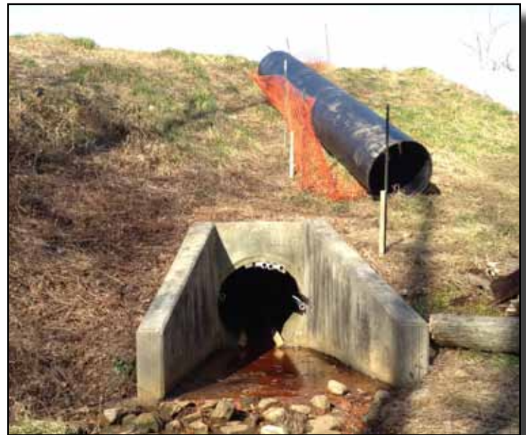
Snap-Tite pipe will be slid inside the old culvert during the installation process.
