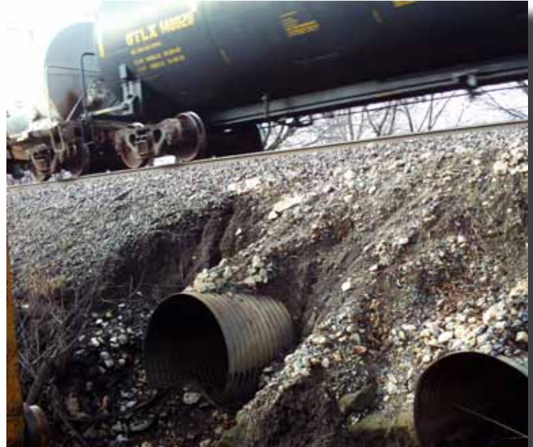
The corrugated metal pipe culverts were in bad shape and needed to be replaced without disrupting the rail service.
