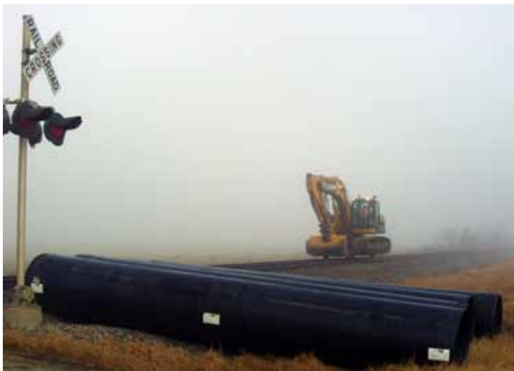
High railing the excavator to the project site. The excavator is used to push the pipe into the culvert.
