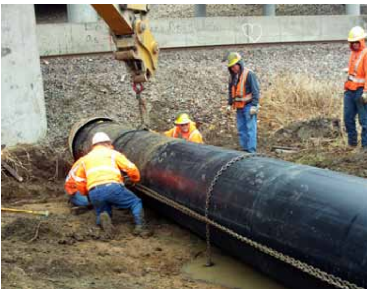
A section of Snap-Tite is pushed inside the old culvert and then snapped together at the machined ends.
