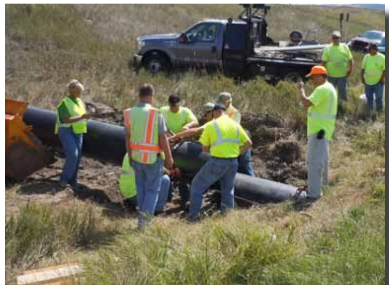
Here observers watch the lining of the 30-inch CMP with 24-inch Snap-Tite pipe.
