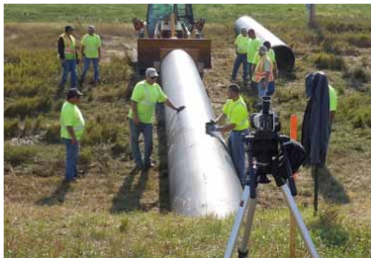
Observers at the demonstration watch the 40-inch Snap-Tite pipe get inserted into the 42-inch CMP.
