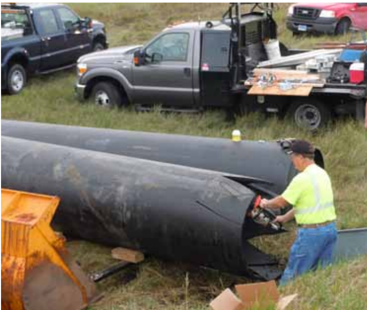
A "bullet nose" is cut on one end of the pipe liner in order to push it easily into the misshaped and damaged culvert.
