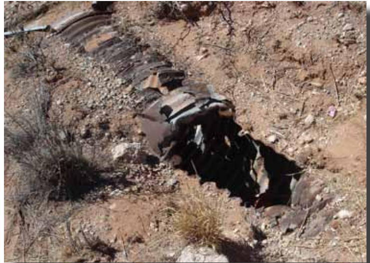
One of the deteriorated culverts underneath SR 31. This one is severely rusted and eroded on top.
