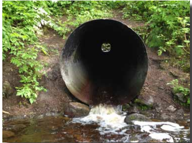
One of the deteriorated culverts.
