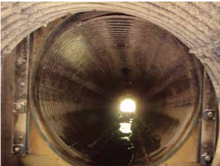
Parts of the old culvert were collapsing. Repair was essential to prevent flooding.
