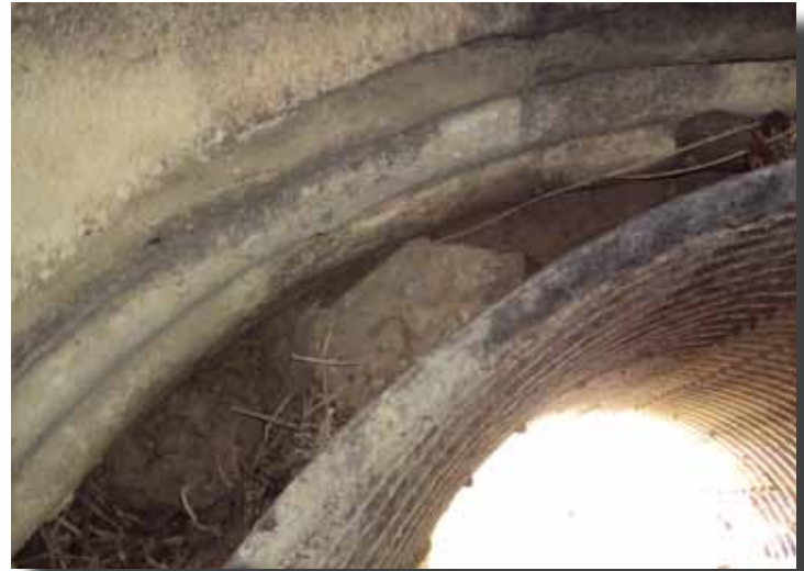
The old levee culvert was damaged and failing in several areas of the length of the pipe. Flooding was a concern.
